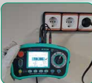
Loop test from a wall socket
